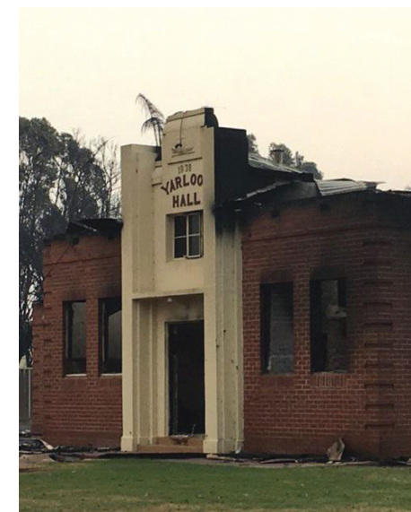
Damage to Yarloop Hall after fire. Credit: Murray Cowper, abc.net.au/news
